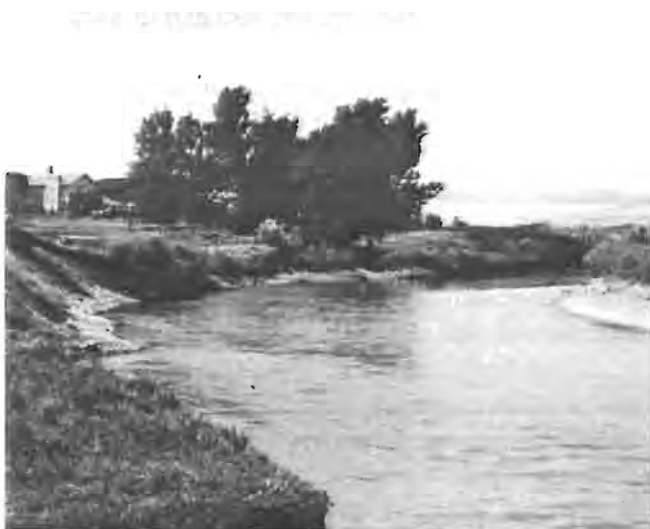
FIGURE 4-3. Channelization of the river bed has caused head cutting, bank collapse and loss of valuable riparian wildlife habitat.
